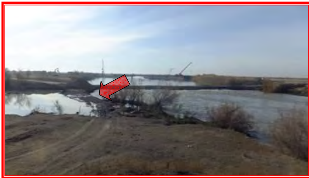
Photo No. 2 : Filter berm is too low and needs to be increased in height
