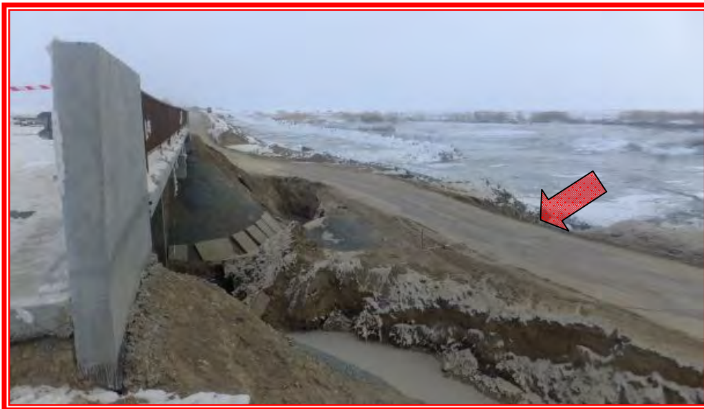
Photo No. 10 : Still the same condition of the narrow crossing at bridge no. 2
