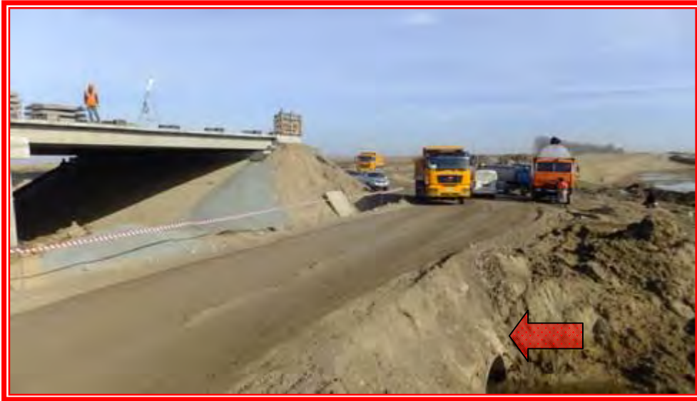
Photo No. 9 : Too narrow diversion crossing at bridge no. 2
