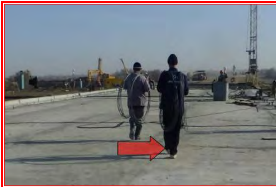
Photo No. 6 : Improper protection by wearing rubber shoes in the work site
