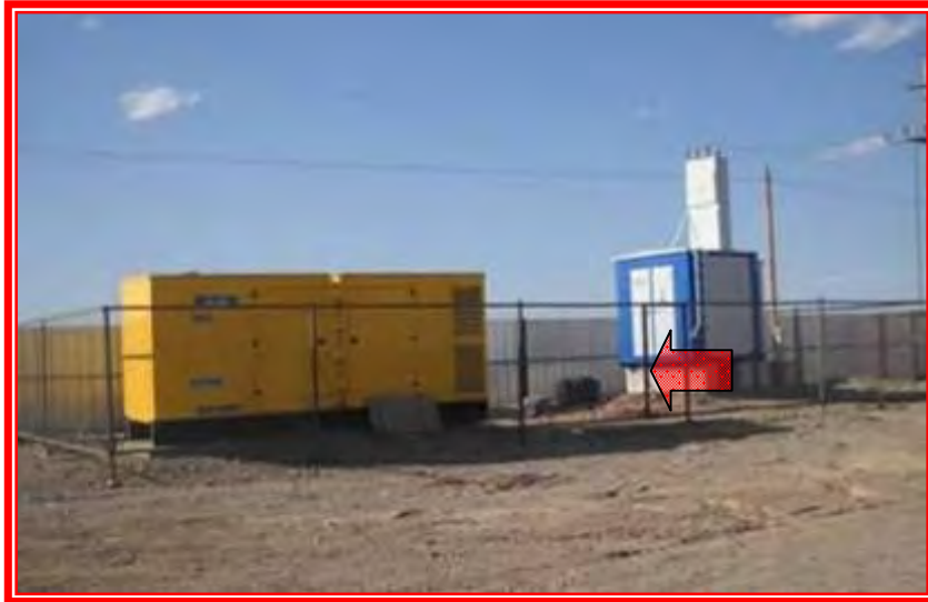
Photo No. 15 : Absence of delineation for safety and absence of warning sign
